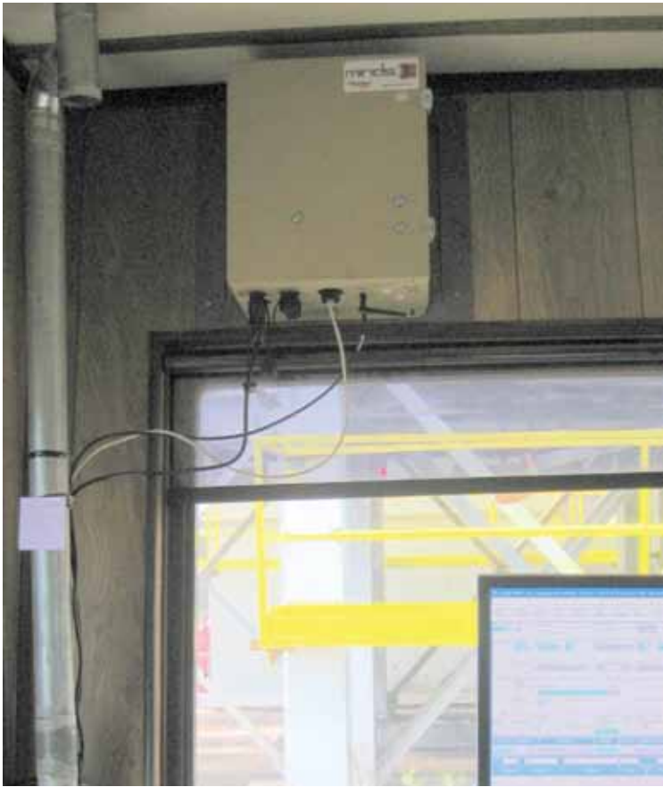
This is the PaveTag box installed inside the control house at SpecAgg.
