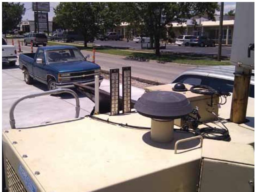
The top of this Lafarge paver includes a marker loop antenna and long range antenna on a jobsite in Wichita, Kan
